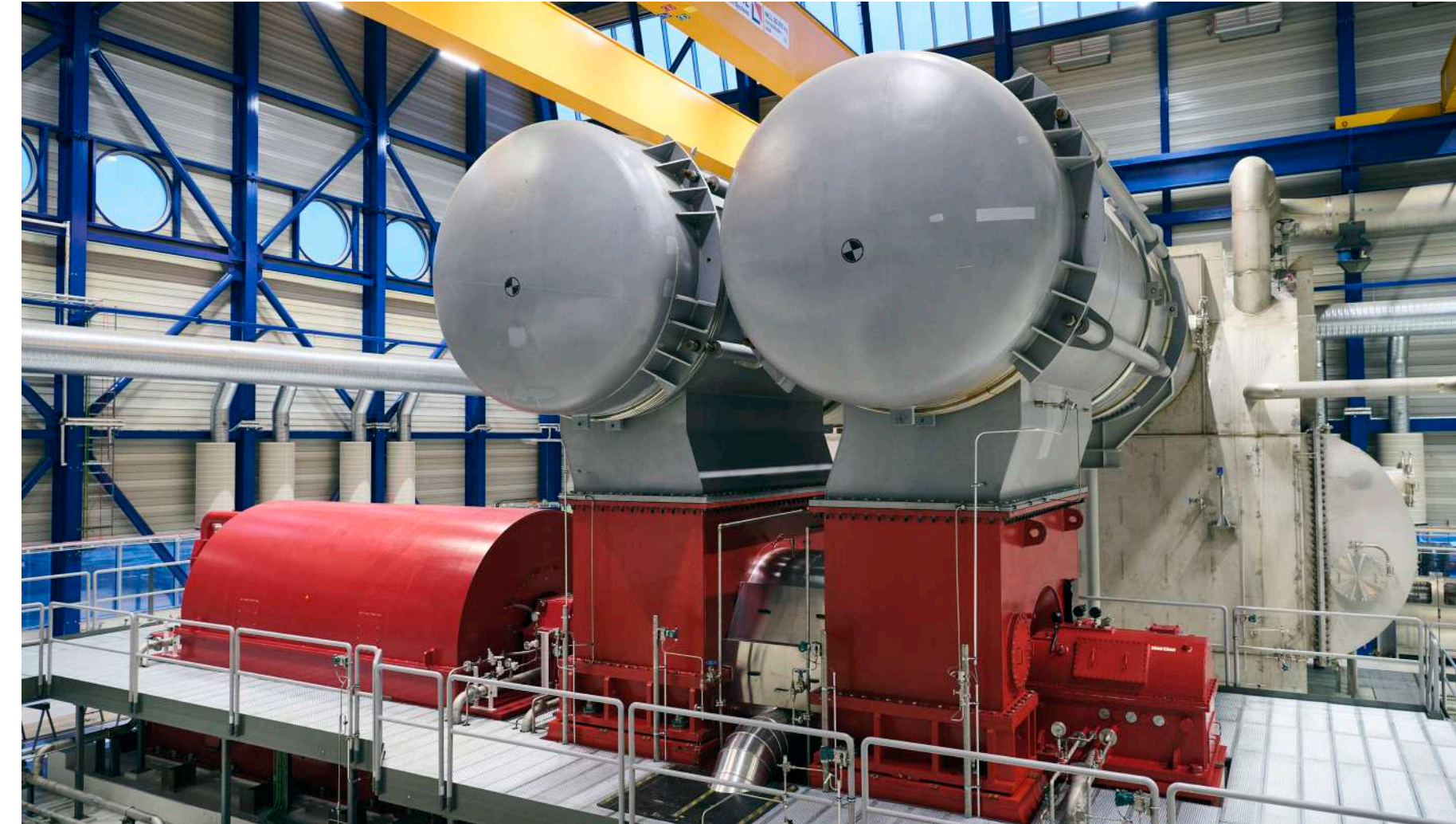
Steam turbine in Svartsengi Power Plant, now the most powerful steam turbine in the country.
