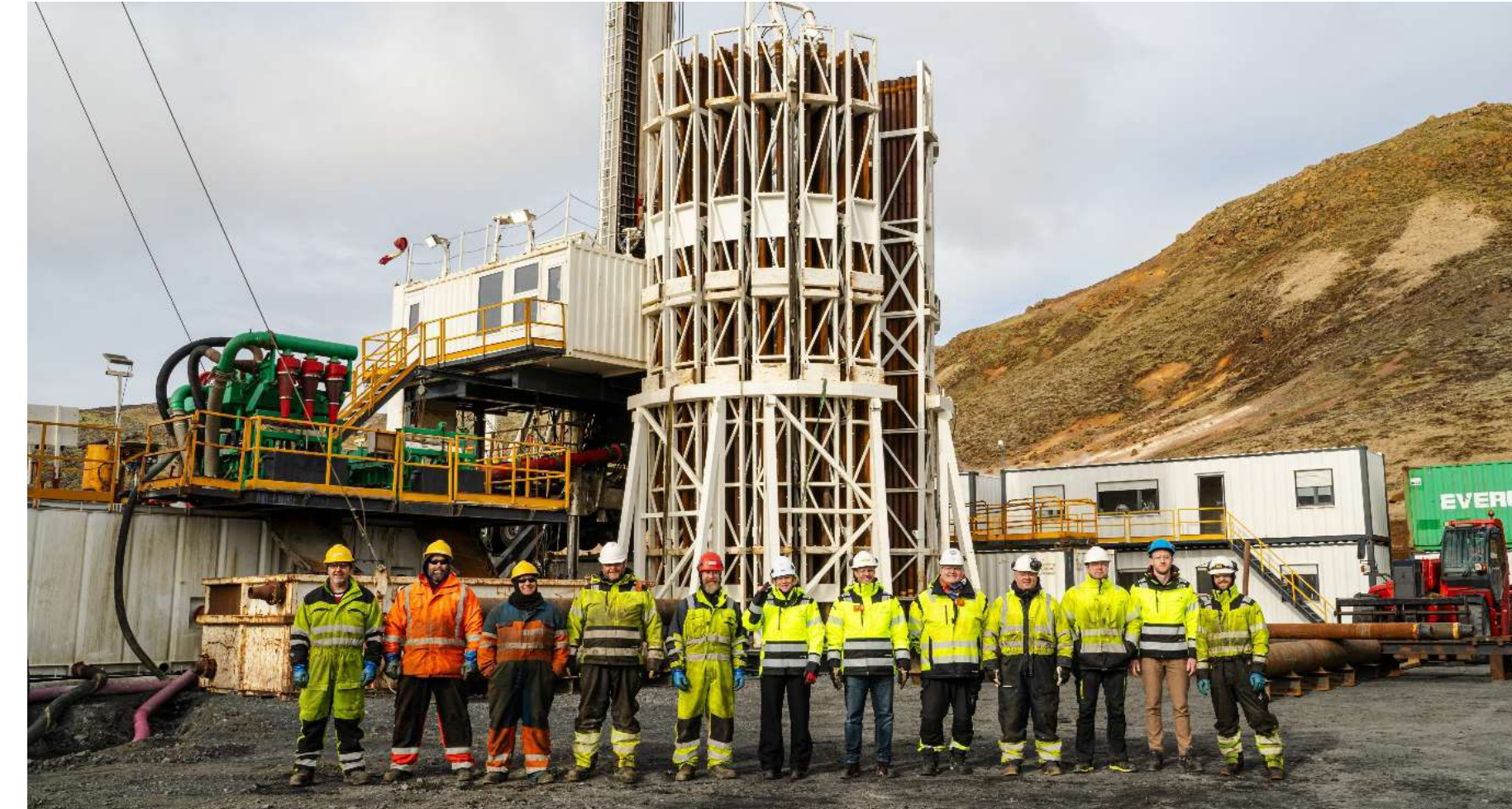
Employees of HS Orka and Jarðboranir on site in 2025 during drilling in the Krýsuvík area.
